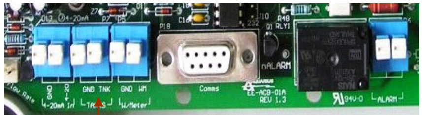
Terminals for Tank Alarm
